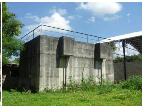
Figura 1.10 – Reator UASB inoperante
